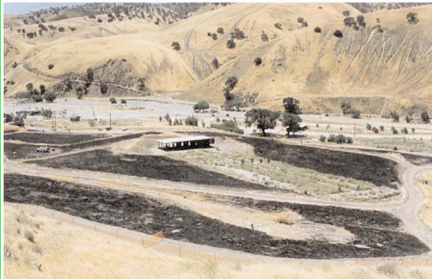
Pit 6 Landfill and overlying rifle range prior to cap construction; view looking south (May 1997).
